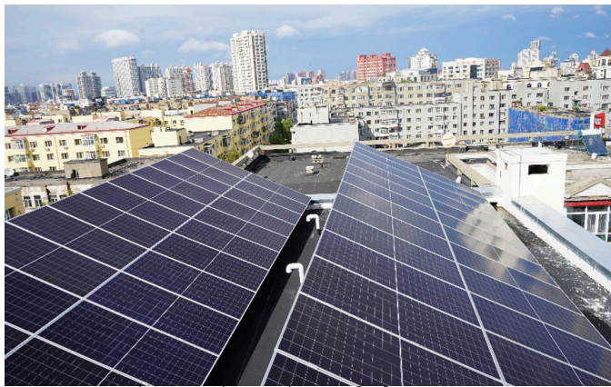
Figure 12: Solar panels on the roof after renovation, source: Harbin DP
