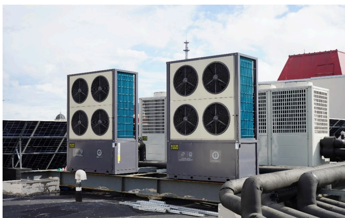
Figure 14: Air-source-heat pump on the roof after renovation, source: Harbin DP
