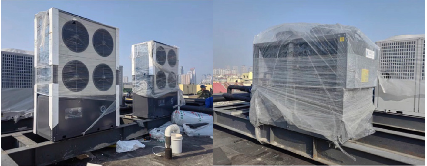
Figure 5: Air-sourced heat pump on roof, Source: Project Presentation 21.12.2023
