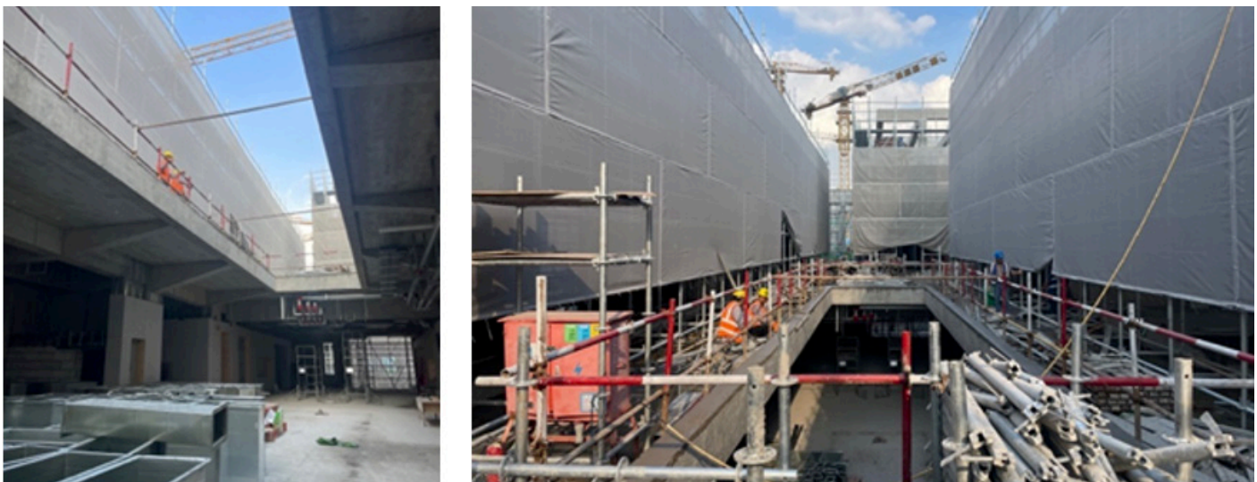
Figure 8: The exhibition hall is under construction. Source: Onsite visit 23.10.2023, ©Sino-Swiss ZEB Project
