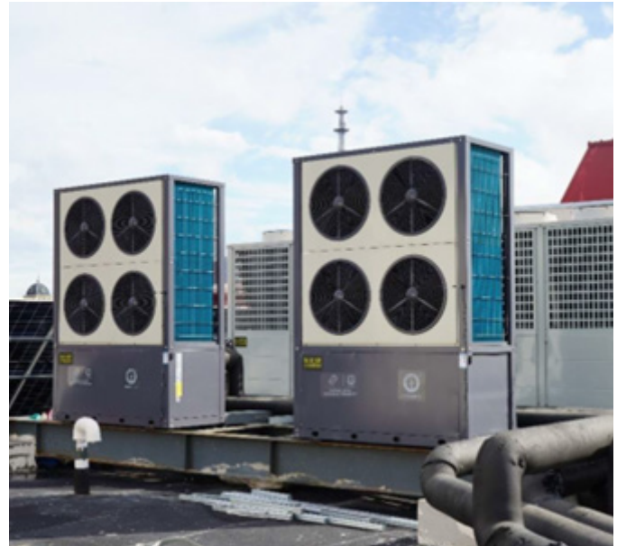
Figure 22: Air-source-heat pump on the roof after renovation, Source: Heilongjiang Cold Land Building Science Research Institute
