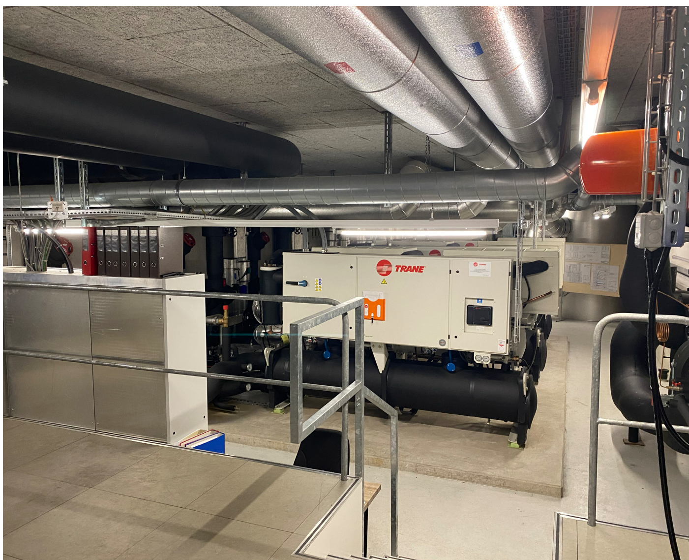
Image: Anergy network system at the Frielager district, Zurich.
