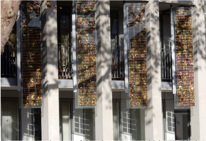
Figure 5: Shadowing of PV elements should be avoided © Kingsgate House, London / P. Bonomo
